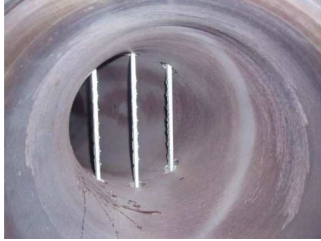
Fig. 3: Thermocouple installation in cold leg elbow section
