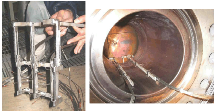
Fig. 4: Thermocouple installation in downcomer (left) and downcomer view from cold leg (right)
